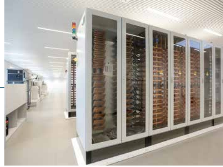
Low Voltage Grid Lab
