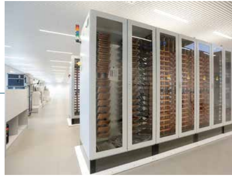
Low Voltage Grid Lab
